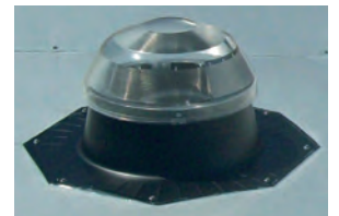
No pitch for over flashing
